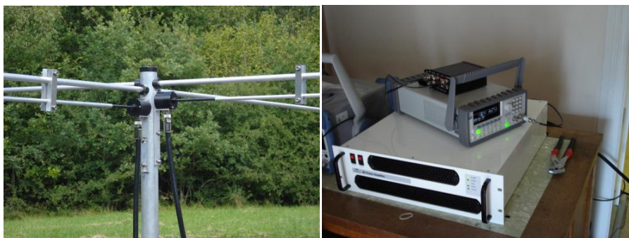
Figure 7 Antenna Elements & Tx Equipment
