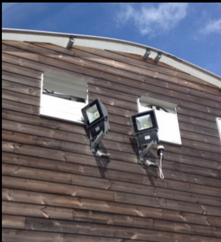
Car park floodlights in a rural area. Nearly half their emissions end up in the sky and surrounding countryside (Photo CfDS)
