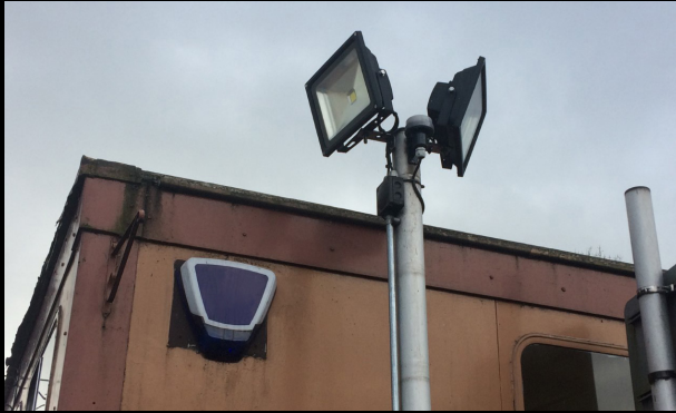
Area floodlighting causing stray light, some of which dazzles drivers on the road beside which it stands
