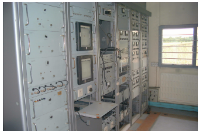
The main control room of the 4C Array.
