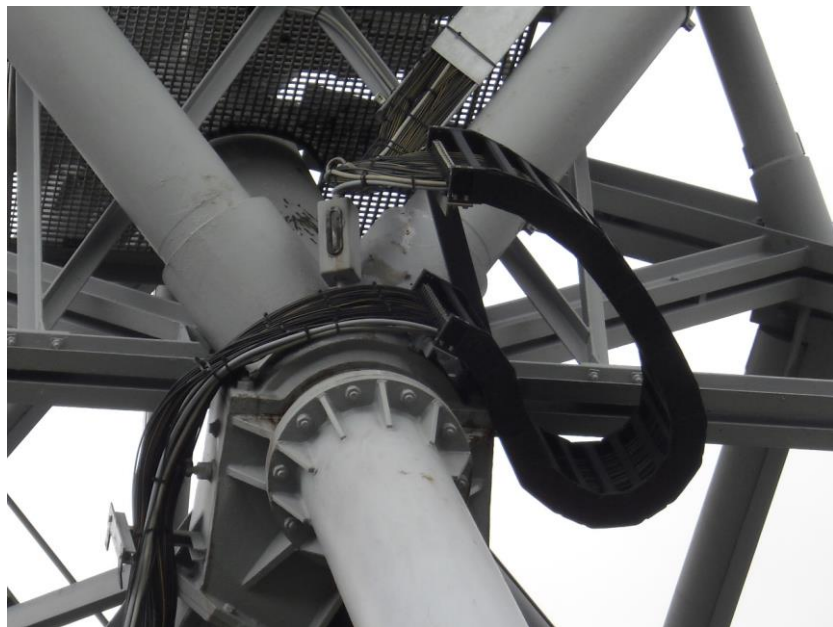
(Figures 5a and 5b Drive and cable management arrangements at each of the dishes)
