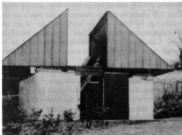
Waterfield's Woolston Observatory after the installation of the new metal clad roof, viewed from the west. (M. J. Hendrie)
